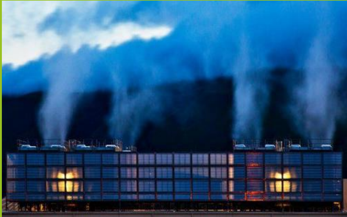
Kühltürme in Google's Rechenzentrum in The Dalles, Oregon
