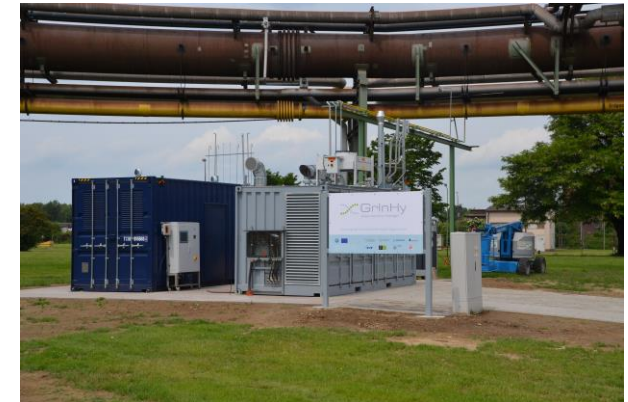
150 kW SOEC module in Salzgitter, Germany
